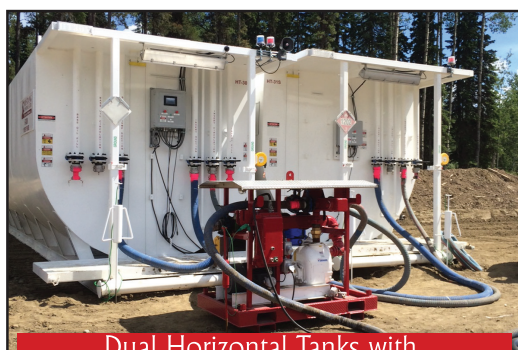
Dual Horizontal Tanks with Remote Pump Manifold
